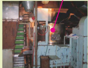
8. oil is drained by a centrifuge
